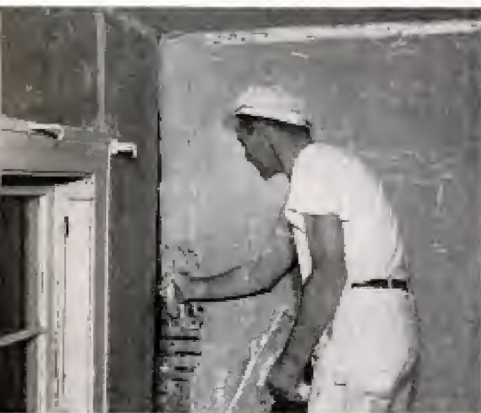
Break in wall is repaired same as ceiling, leveling with float. Roughened surface on plaster formed by float or darby is needed for finish-coat adhesion
